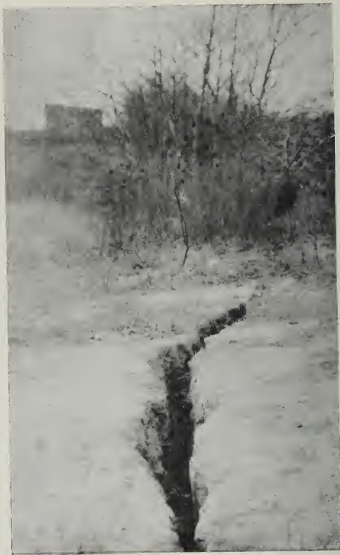
FIG. 8.—Crack, 8 to 10 inches wide, due to subsidence over the north panel shown in figure 7. The view was taken from A looking west. (Photo by J. R. Fleming, U. S. Bureau of Mines.)
